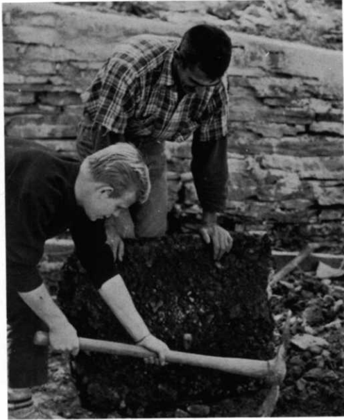
Brother Vincent employs the help of many students in his various projects. Here Brian Bonner prepares the groundwork as Brother waits with a slab of concrete.
