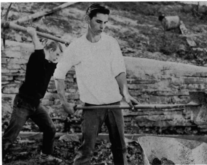
Tom Zwolinski and Brian Bonner are hard at work as they prepare a bed for the new sidewalk.
