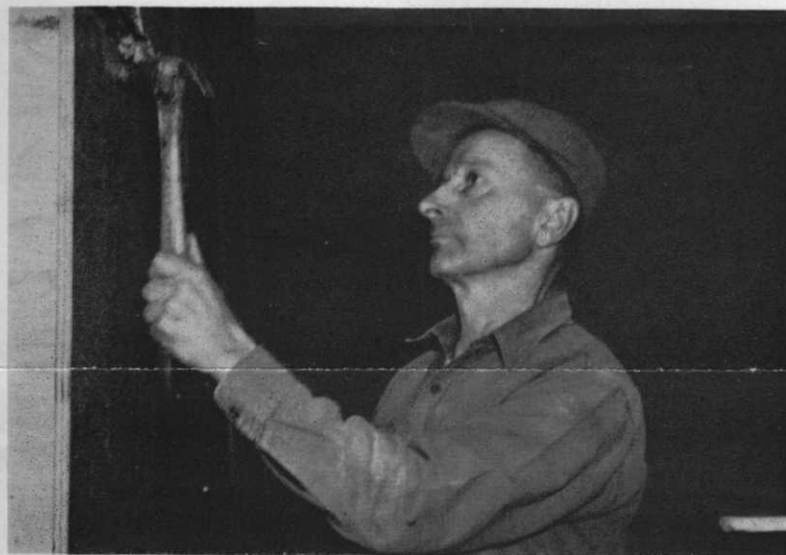
Mr. Johann Grych, our master carpenter and craftsman, working on the remodeling of one of the classrooms
